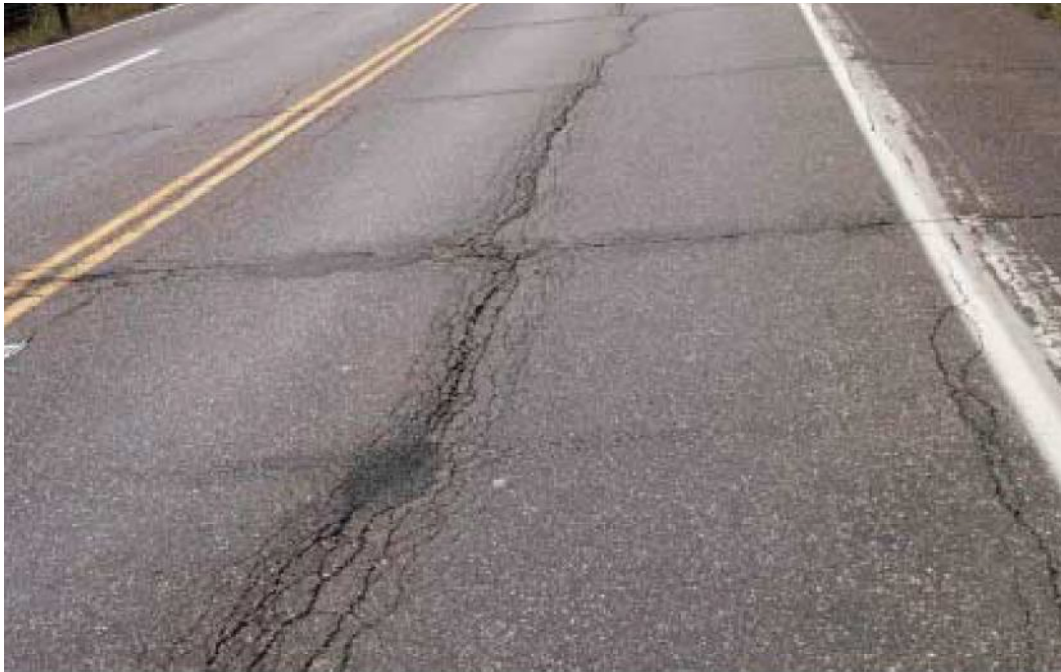
Figure 3.1. High severity longitudinal and transverse cracks.
