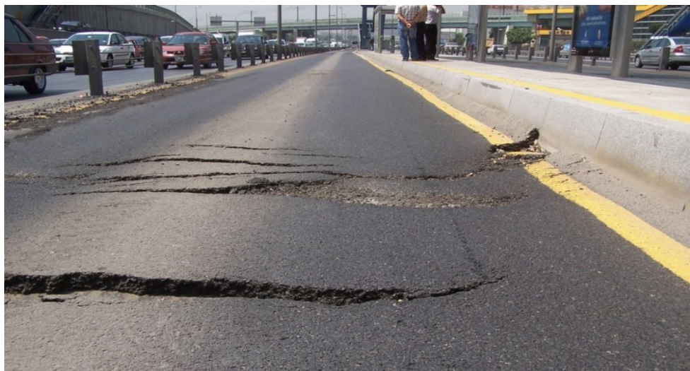
Figure 7.4. Permanent Deformation on METROBUS Line Surface
