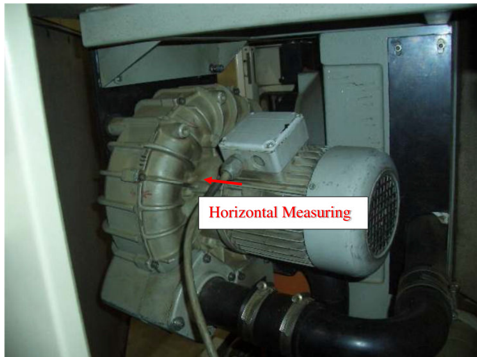
Figure 5.5: Motor-fan mechanism horizontal measuring.
