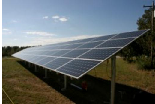
Figure 4. 27 : Solar Photovoltaics ( http://greenliferetreats.com ).
