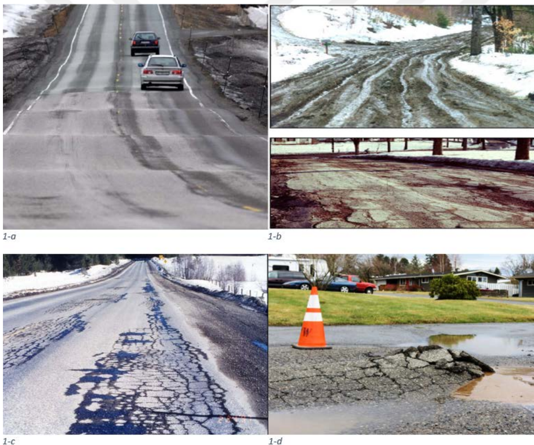
Figure 2.1 : Visual Signs of Pavement Damage Caused by Freeze-Thaw Cycles: (1-a) frost heave in Norway (Ystenes, 2011), (1-b) thaw weakening on an unpaved road (Shoop et al., 2008), (1-c) alligator cracking ("Frost Action,"), and (1-d) frost boils on an asphalt road ("Frost boils – the reason for emergency road restrictions | Whatcom News," 2017).
