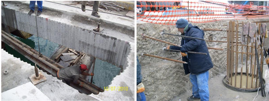
Figure 4-36 Making the base mold, pouring the pile concrete and planting sprouts with epoxy
