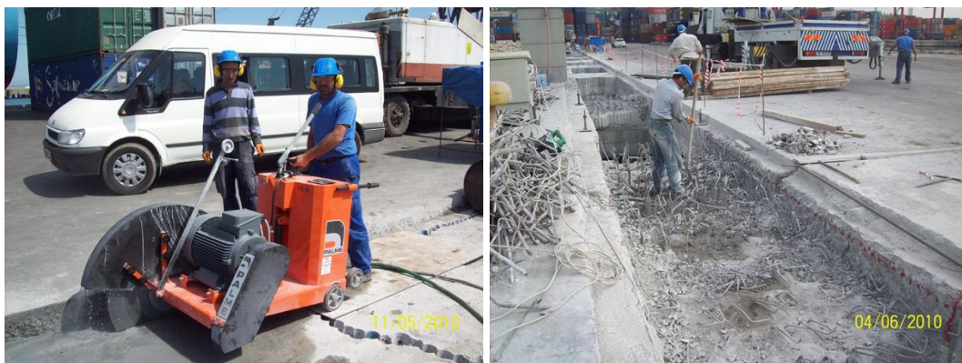
Figure 4-33 Cutting the designated area to a depth of 10-15 cm using a grooving machine and clearing away the debris
