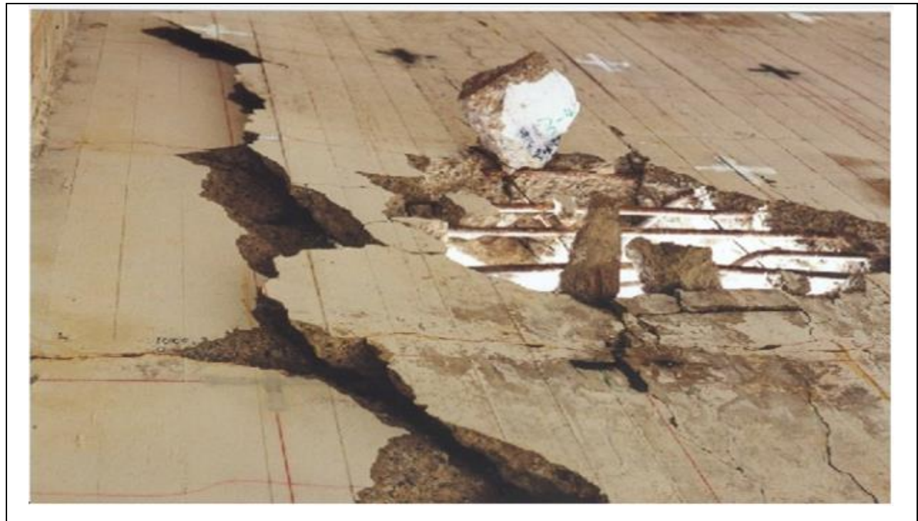
Figure 1.1: Punching Shear Failure in a Bridge Deck
