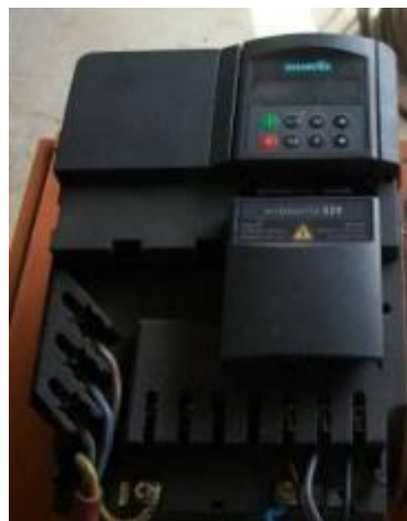
Figure 4.2. Siemens frequency converter.
