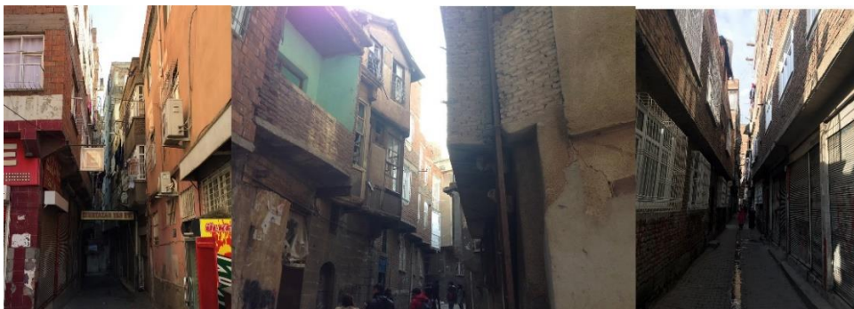
Figure 26 Distortion on Physical Structure of Houses. (METU MUD, 2017)
