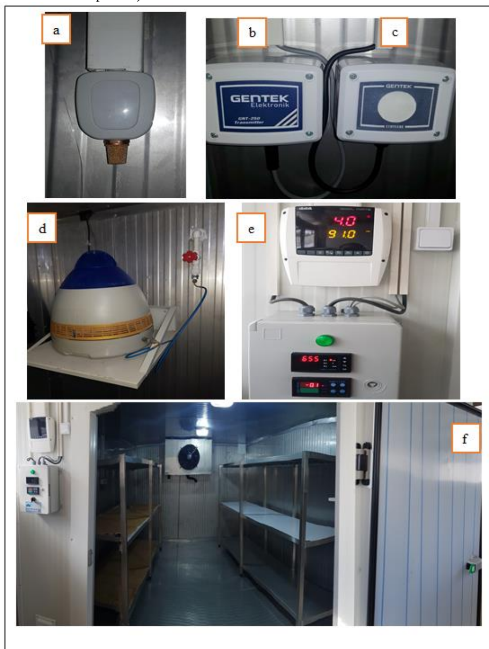
Appendix 20. Description of the cold room. a) humidity sensory, b) CO 2 sensor, c) ethylene sensor, d) Cezio humidifier device, e) Digital control panel f) overall view of cold room
