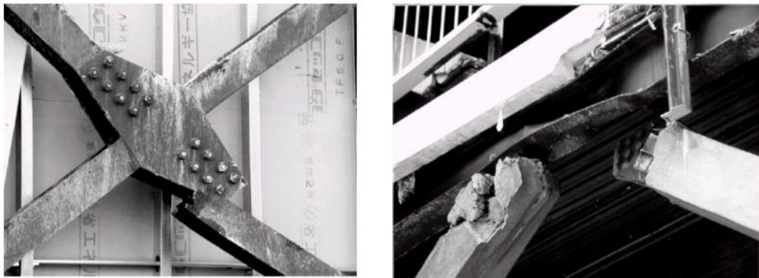
Figure 2.11 Damage to nonductile braces in Kobe earthquake: net fracture at bolt holes (left) and severe distortion of unstiffened beam in chevron braces (right) (Naeim, 2001)
