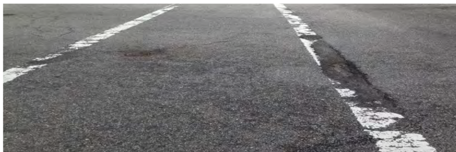
Figure 2.7 Example of Poor Maintenance of Road Markings
