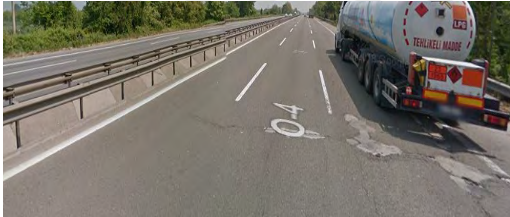
Figure 4.8 Example of Anatolian Highway/ Poor Road Surface
