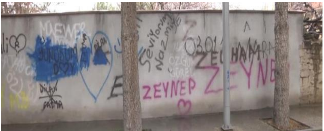
Figure 3. 7. The Wall of Tahir Hodja's House Previously (Konhaber, 2016)
