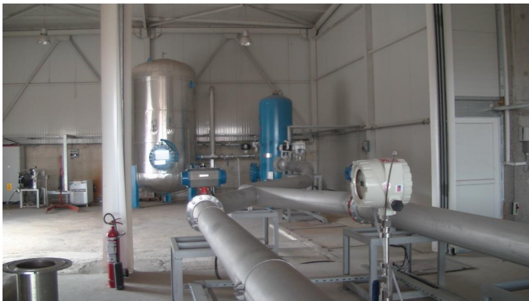
Figure 4.6: Compressed dry air system with thermal mass flow meter.
