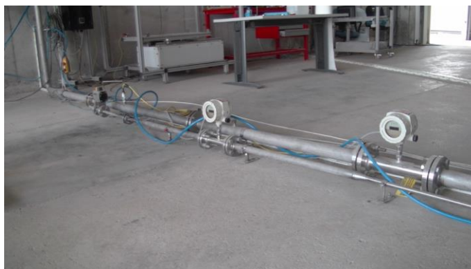
Figure 4.27: Thermal mass flow meters located on oxygen replenishment and pilot oxygen lines.
