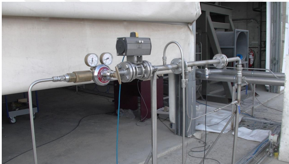
Figure 4.12: Fuel supply line with its instrumentation.
