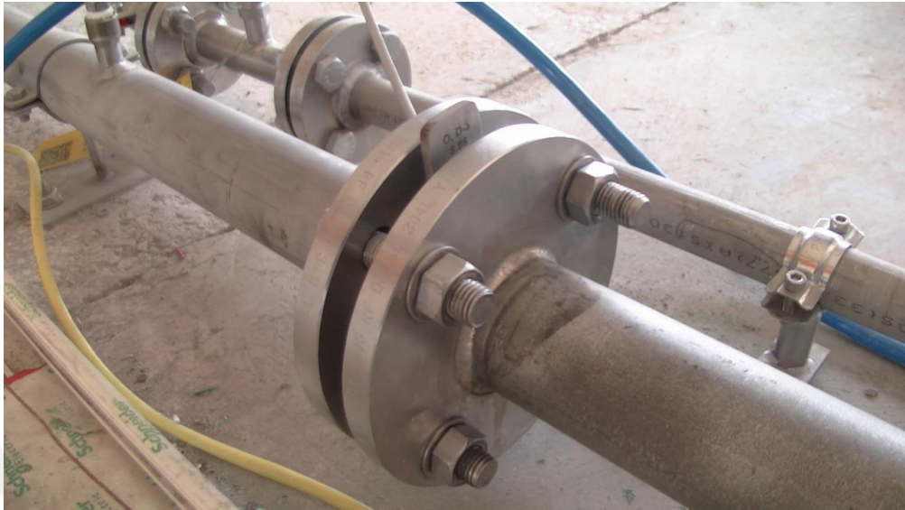
Figure 4.10: Orifice plate placed on the oxygen replenishment line.
