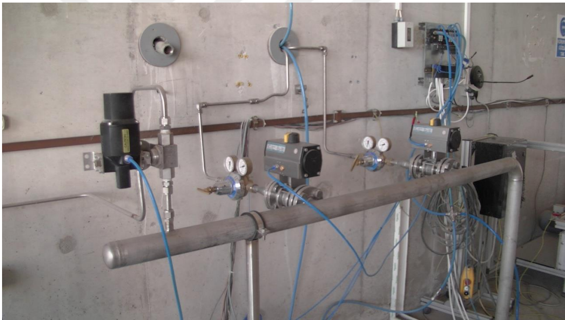
Figure 4.7: Shut-off valves and pressure regulators of the oxygen replenishment line.
