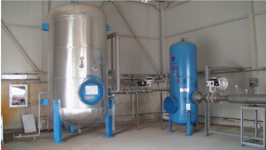
Figure 4.5: Compressed dry air system.
