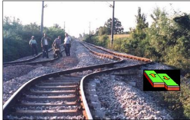
Figure 2.7. Fault displacement after the 1999 Kocaeli Earthquake.
