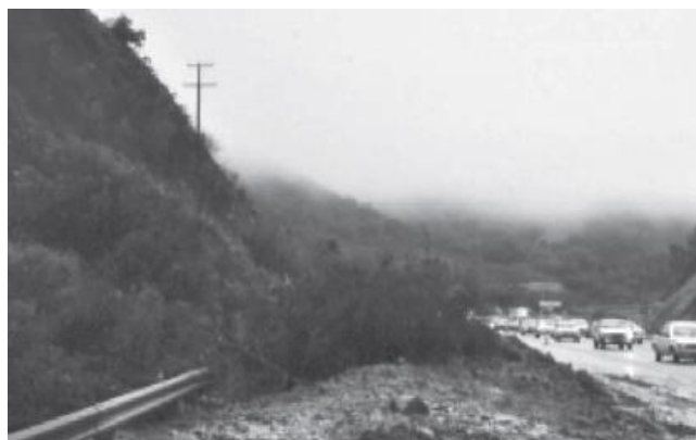
Figure 2.3. Flow slide on Highway 24 (Duncan, 2005).
