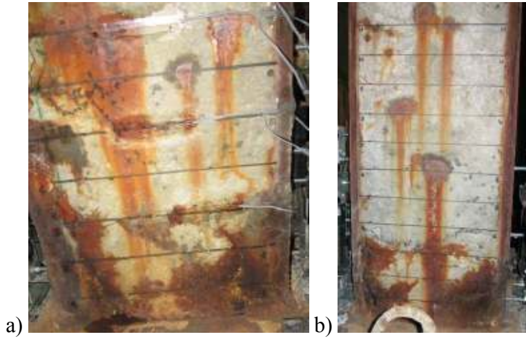
Figure E.277: a) North, and b) South view of NS-X54 after -0.25% drift ratio.
