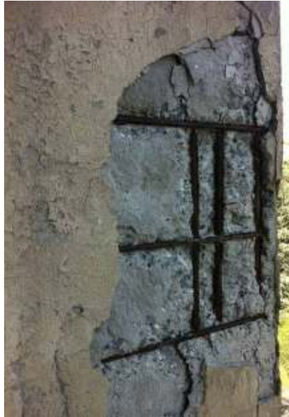
Figure 6.53 : The appearances of existing sub-standard RC frame structures.
