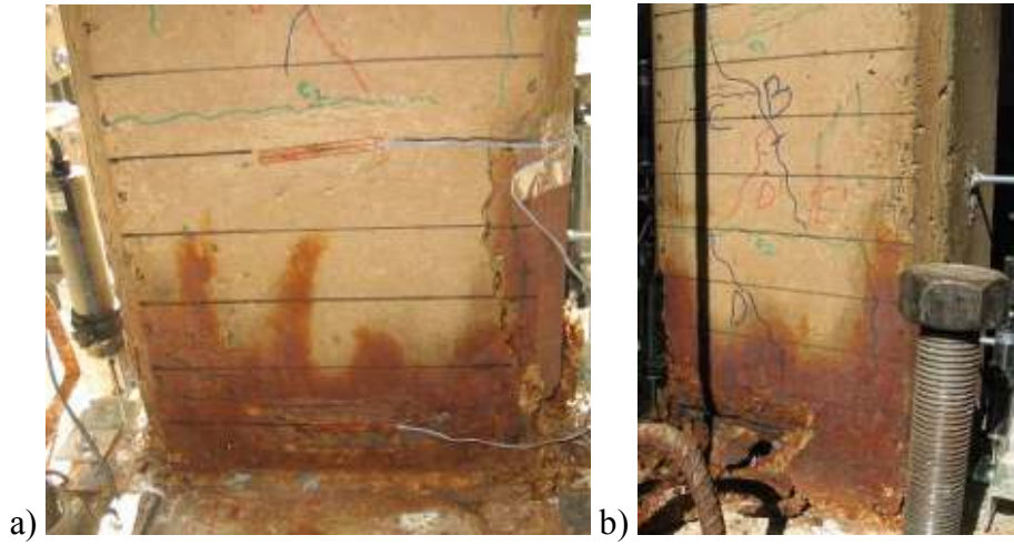
Figure E.135: a) North, and b) South view of LS-X19-H after -3.5% drift ratio.
