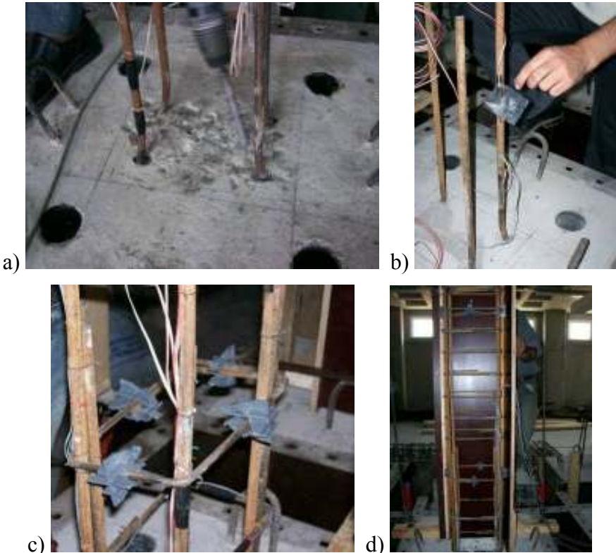
Figure 5.2 : Preparation of columns (a) Chipping at the interface, (b) Bonding strain gauges to the starter bars, (c) Placement of plastic spacers for concrete cover, (d) Placement of molds.
