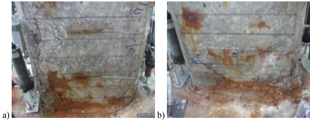
Figure E.263: a) North, and b) South view of NS-X22 after -2.5% drift ratio.
