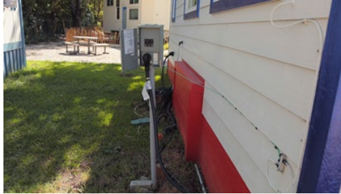
Figure 74. Separate electricity and WIFI (Lantrop, 2022).
