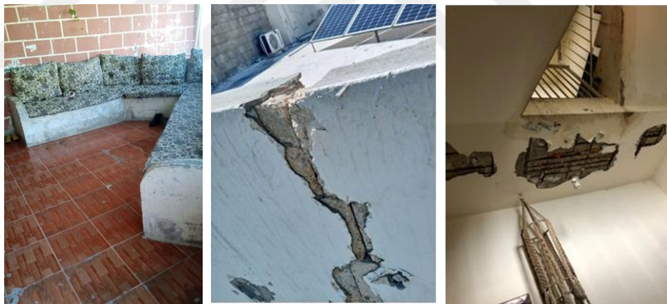
Figure 17. Photographs of structural cracks in some houses in Qalamoun, by author
