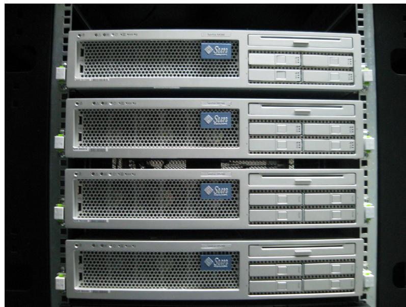
Figure 12. New four node processing server setup
