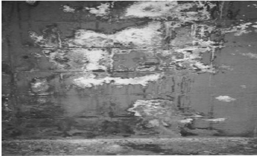
Figure 2.6 Penetration of sulfate-bearing ground water through a retaining wall exposed to atmospheric changes (wetting–drying, heating–cooling)
