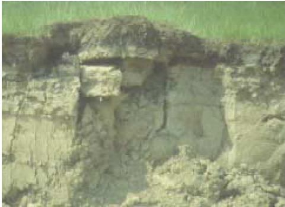
Figure 3.6. Crack in a compacted clay barrier in a landfill cover in southern Wisconsin, USA (Albrecht, 1996)
