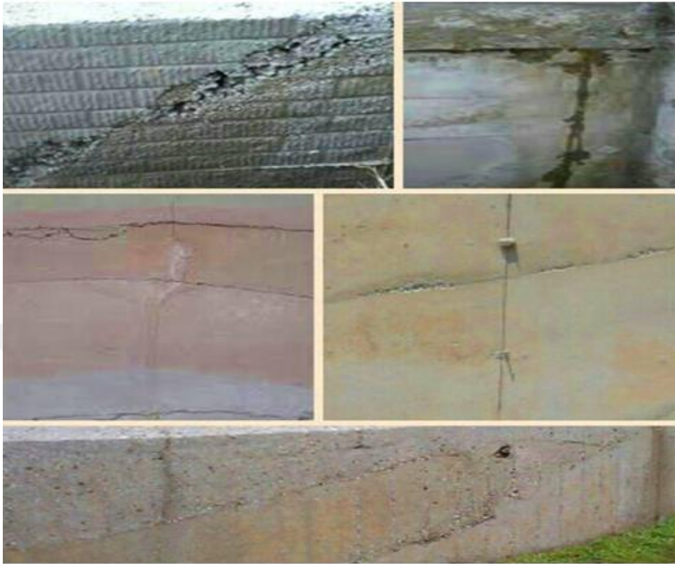
Figure 2.1. Irregular cold joint.
