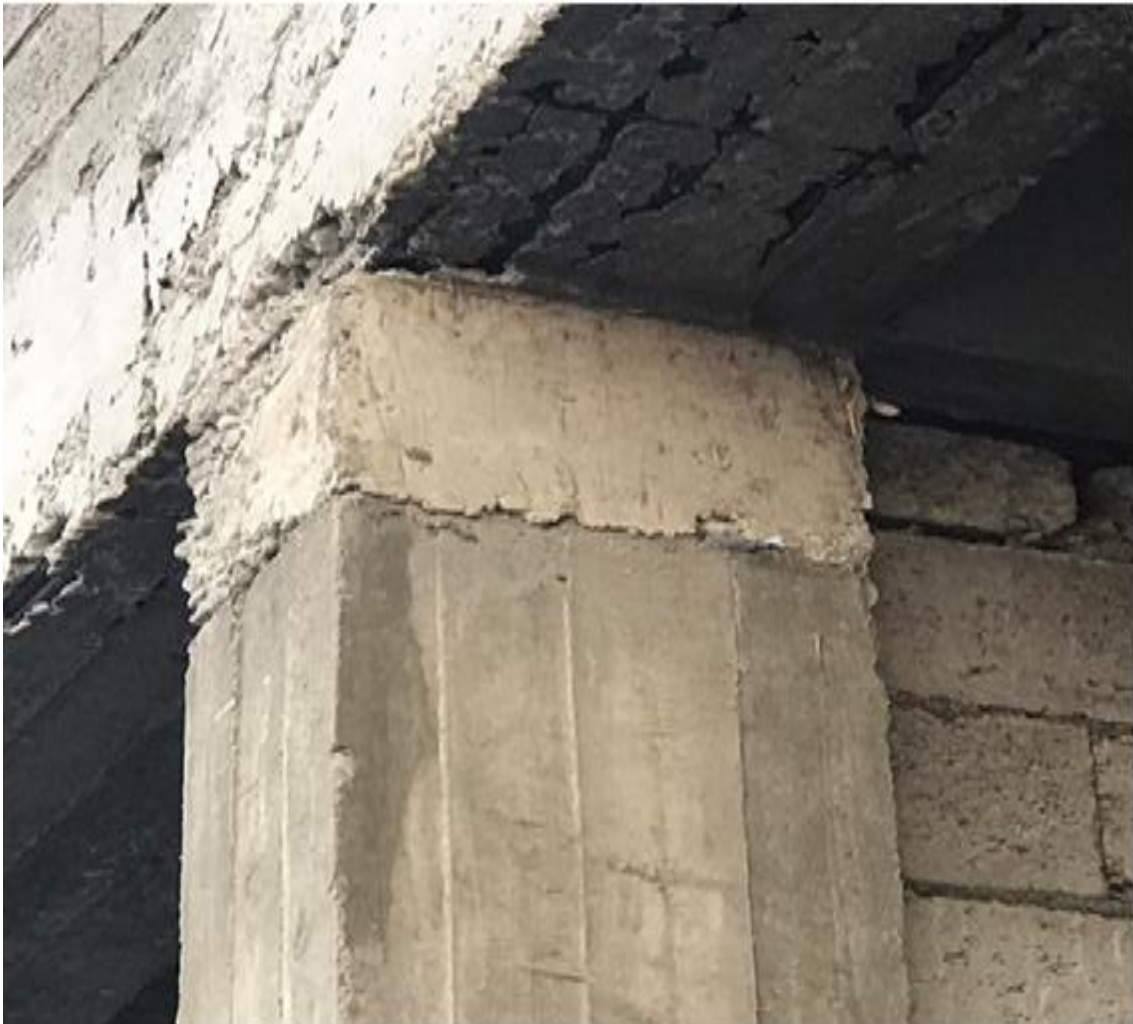
Figure 1.3. Cold joint in a column (Picture from Erbil City 2019).
