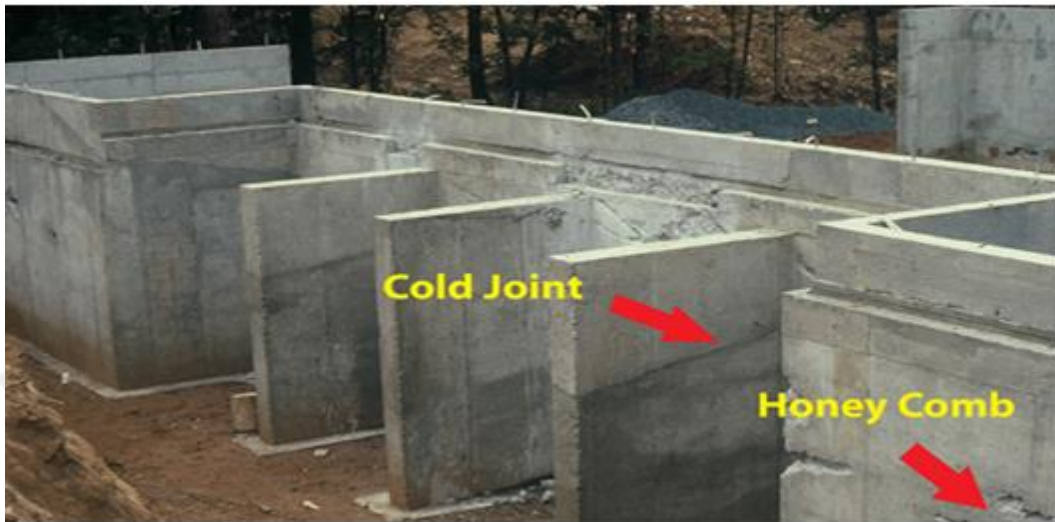
Figure 1.2. Cold joint on wall.
