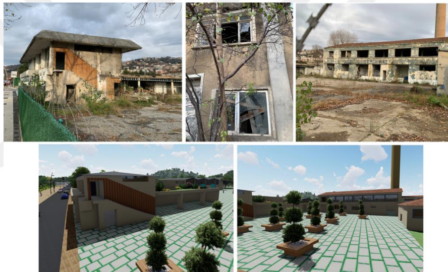
Figure 4.16: Existing situation of the buildings facades and broken windows (Up) and proposed proto-designed image of the buildings and facades (Down).
