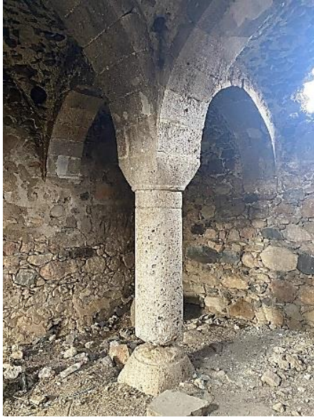
Figure 4.21. Sectional weakenings observed on the columns (Author's Archive, 2023)
