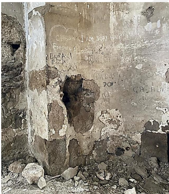
Figure 4.20. Damages observed on walls due to vandalism (Author's Archive, 2023)
