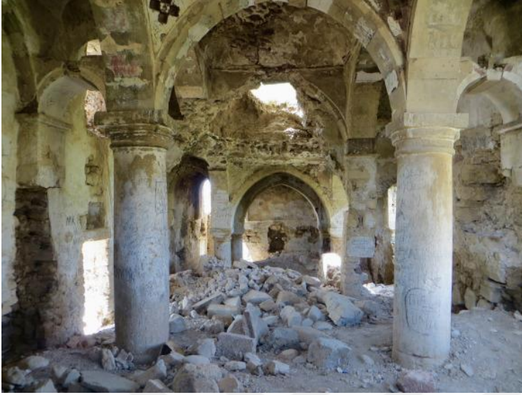
Figure 3.25. Deterioration of the Surp Hulvenk Monastery due to vandalism (Source: https://arkeofili.com/elazigdaki-1000-yillik-hulvenk-kilisesi-10-yildir-tahrip-ediliyor/ , Access Date: 02/11/2023)
