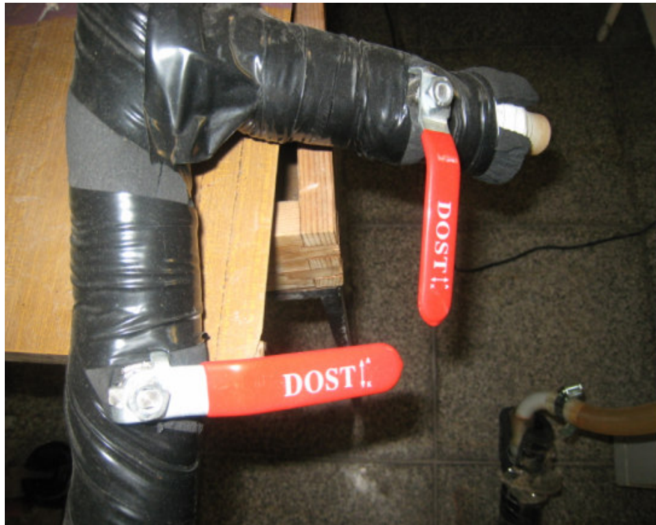
Figure 2.7 Flow rate measurement valve
