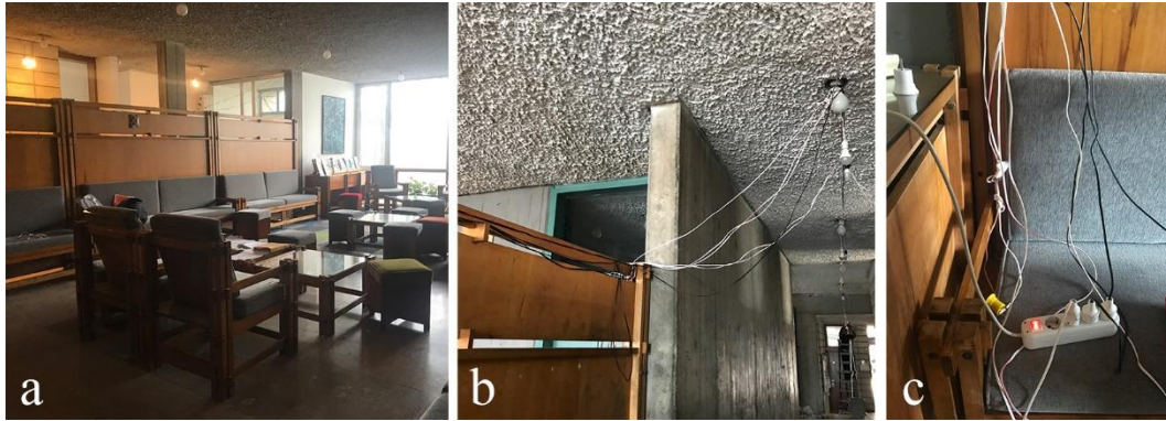
Figure 3.5. Inside of the control room (a), cables going into control room (b), control point in the control room (c).
