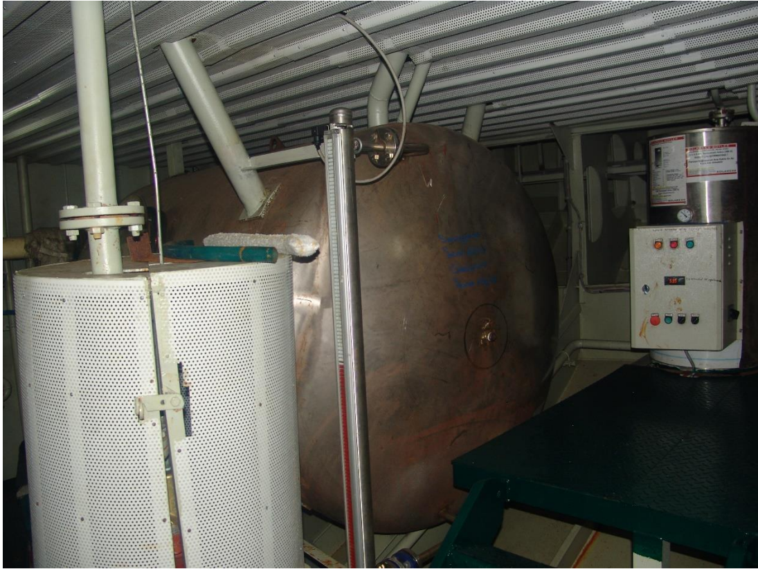
Figure A.13: FM-200 Tank.
