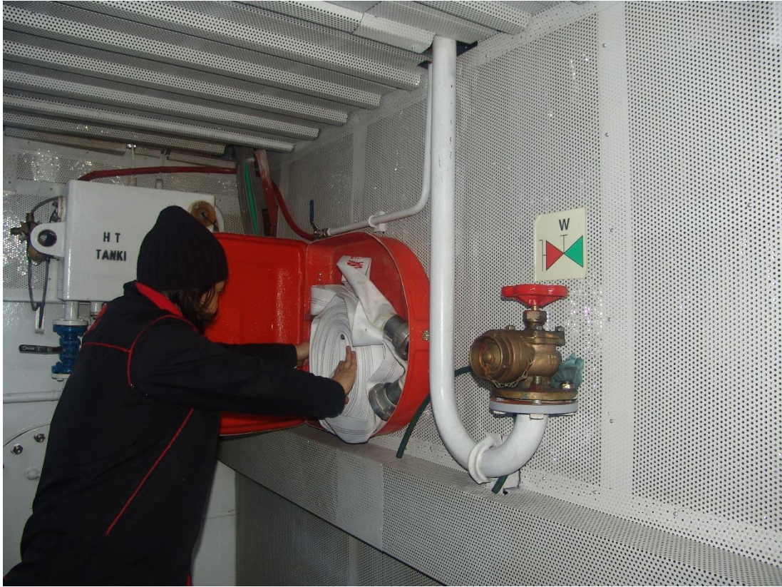
Figure A.11: Fire Extinguishing Hose.
