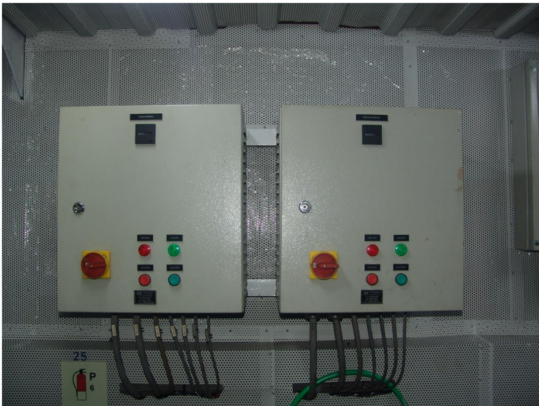
Figure A.10: Fire and Bilge Pump Boards.
