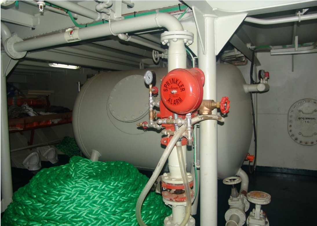
Figure A.2: Sprinkler Alarm System.
