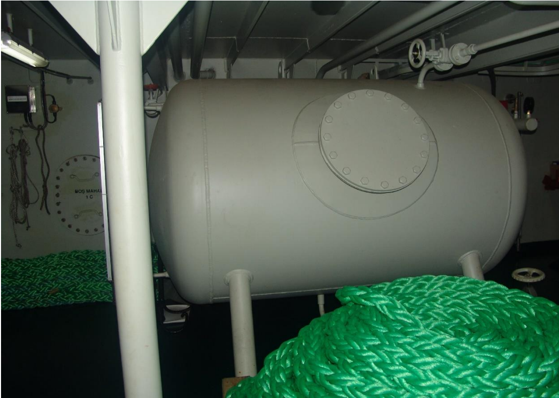
Figure A.1: Sprinkler System Tank.
