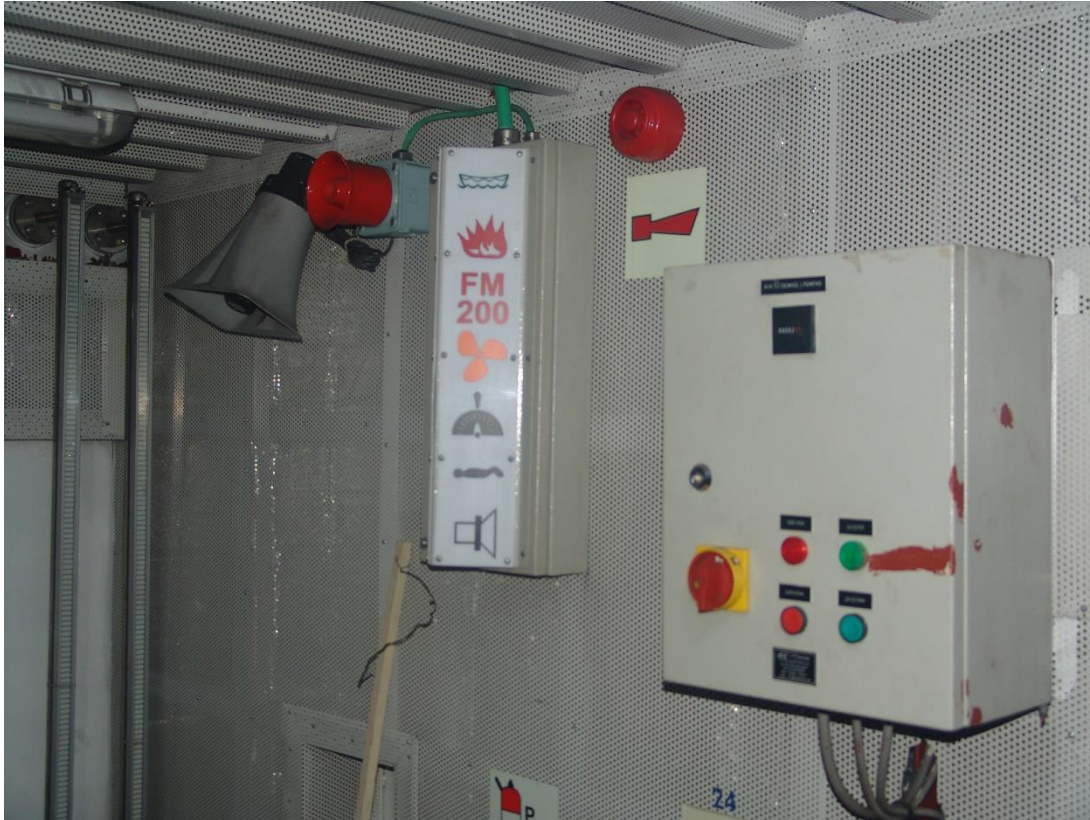
Figure A.9: FM-200 Alarm System.
