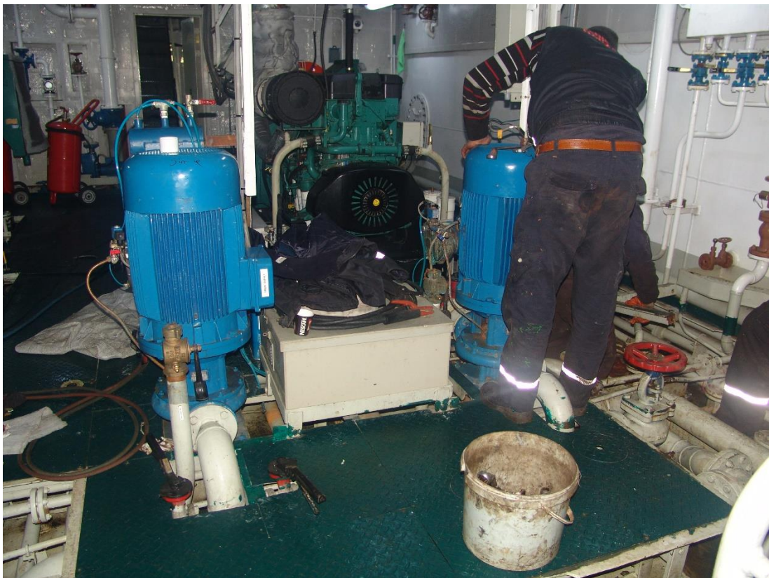
Figure A.12: Fire and Bilge Pumps.
