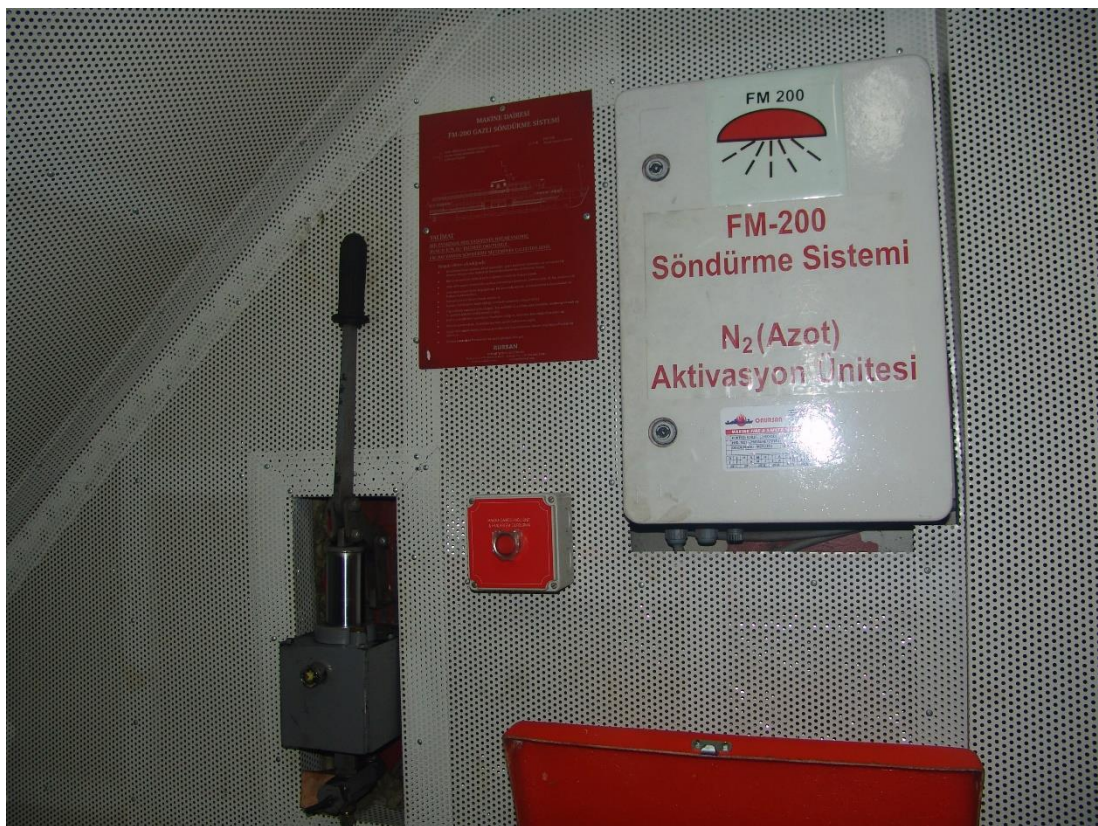
Figure A.4: FM-200 Extinguishing System and N 2 (Nitrogen) Activation Unit.
