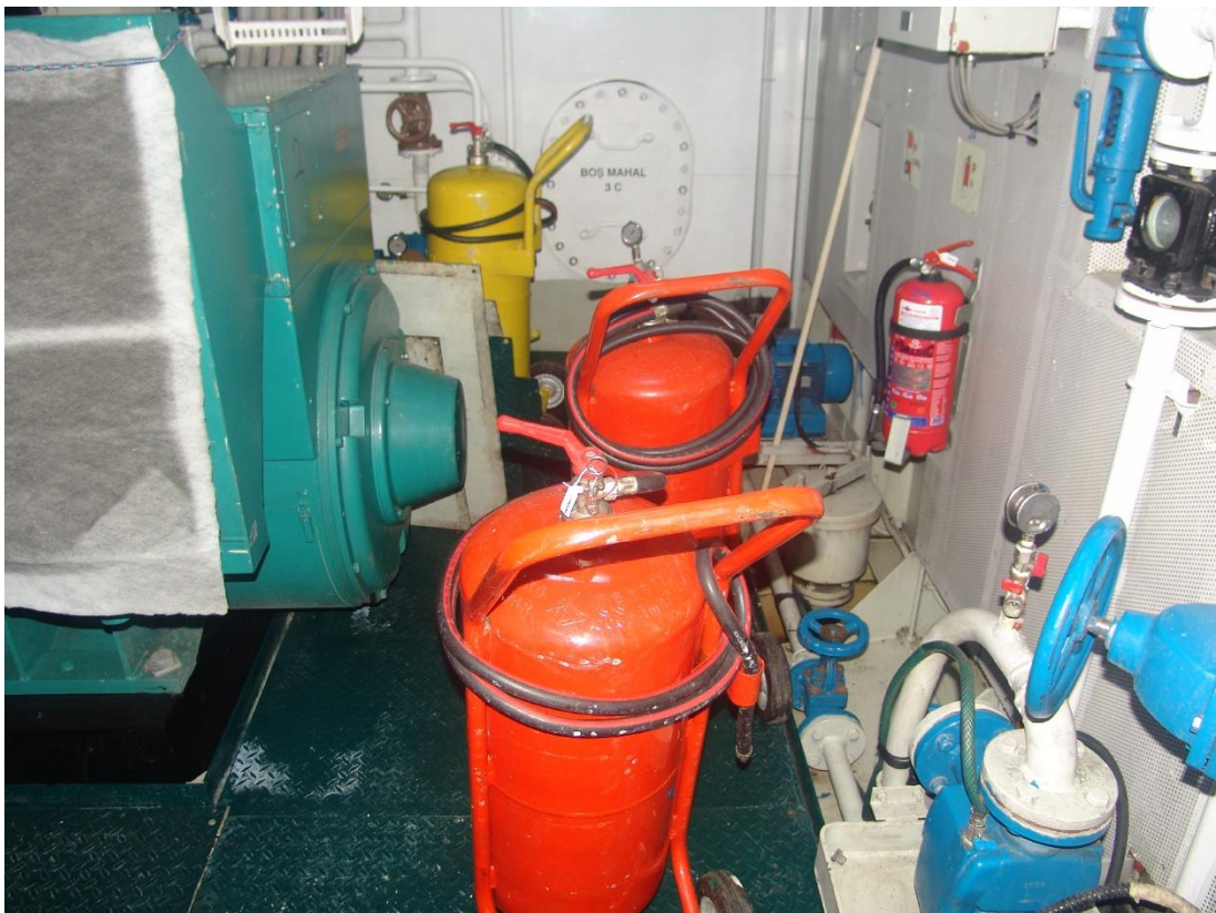
Figure A.8: Portable Extinguishers.
