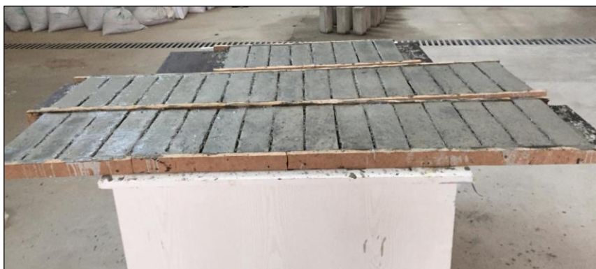
Picture 3.4. The formwork of the small segments before and after pouring the concrete.
