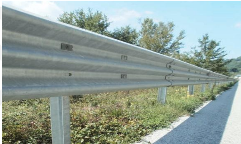
Figure 3.4. Thrie beam guardrail [15].
