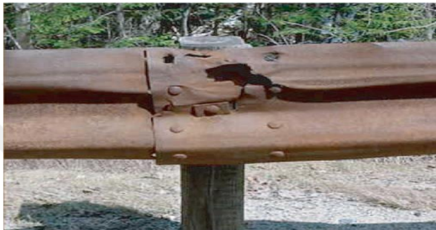
Figure 3.6. Steel beam guardrail deformation [77].
