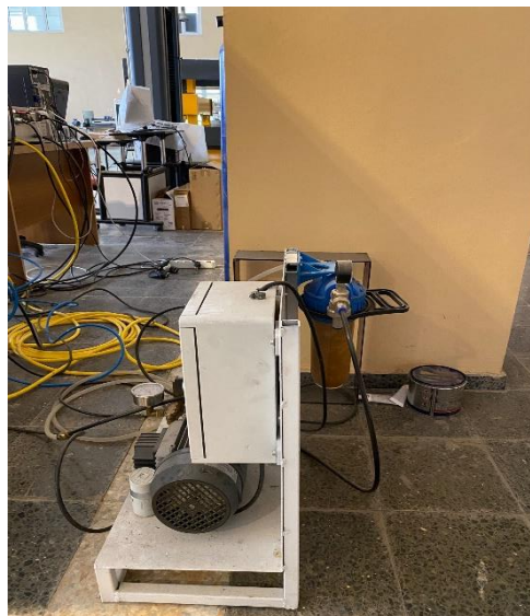
Figure 5.5 Water pump unit with filtration
