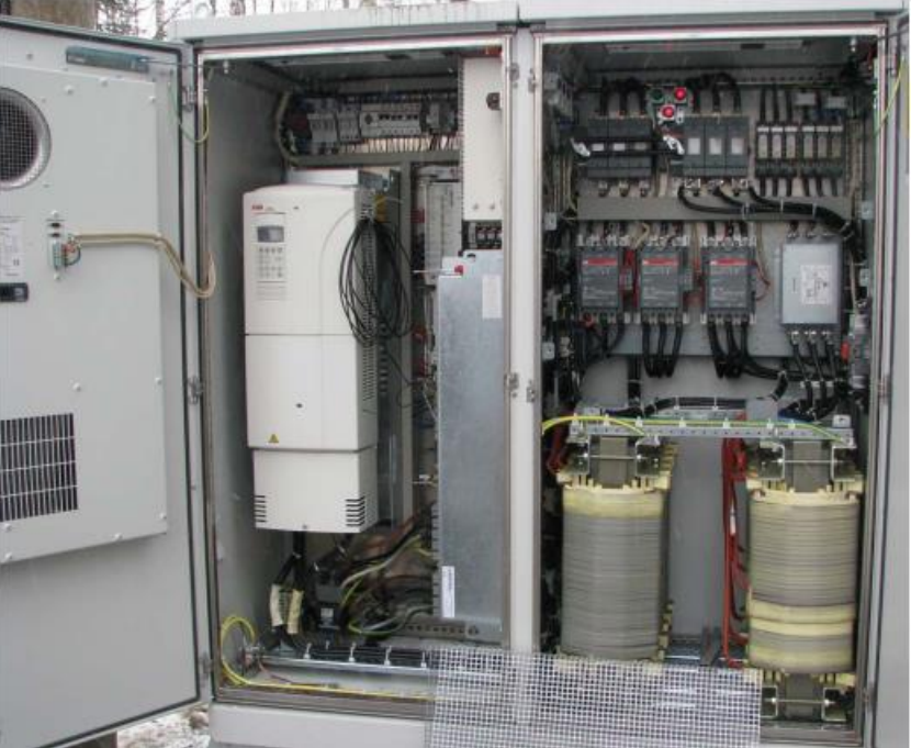
Figure 4.3 : ABB ACS800-11-5 Converter Installation [21]
