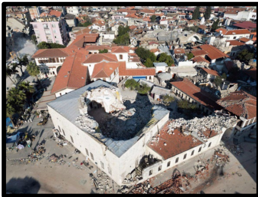
Figure 1.12. Habib-i Neccar Mosque, a masonry structure failed due to earthquakes (top view) [18]
