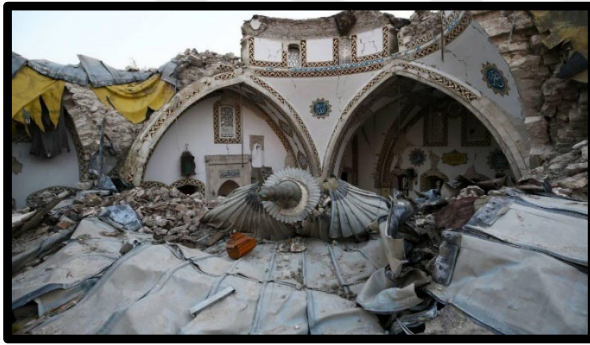
Figure 1.11. Habib-i Neccar Mosque, a masonry structure failed due to earthquakes (inside view) [18]
