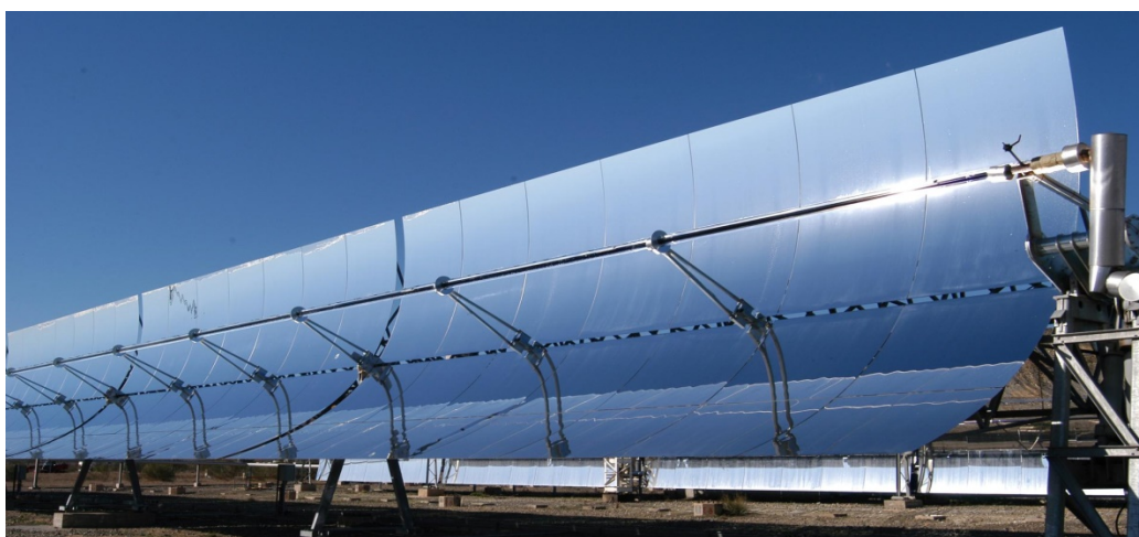
Figure 2.4: Front (left) and rear (right) views of EuroTrough collector [2].
