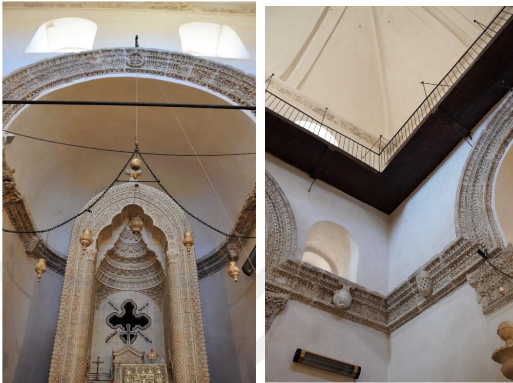
Figures 5.38 and 5.39: The restored interior of the church of Deyrul Zafaran Monastery, October 2019.
