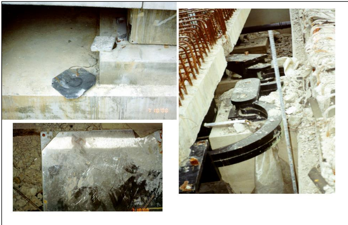
Figure 5.3. Complete failure of existing protection systems of Bolu Viaducts.
