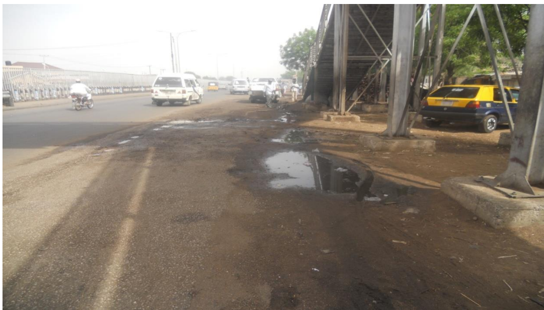
Figure 4.27 Improper pillar location (Km 03+900) Airport Roundabout-Bachirawa Junction
