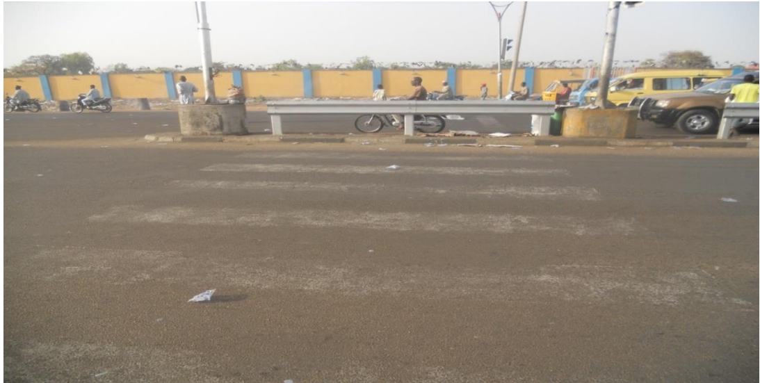
Figure 4.38 Faded and blocked pedestrian crossing
