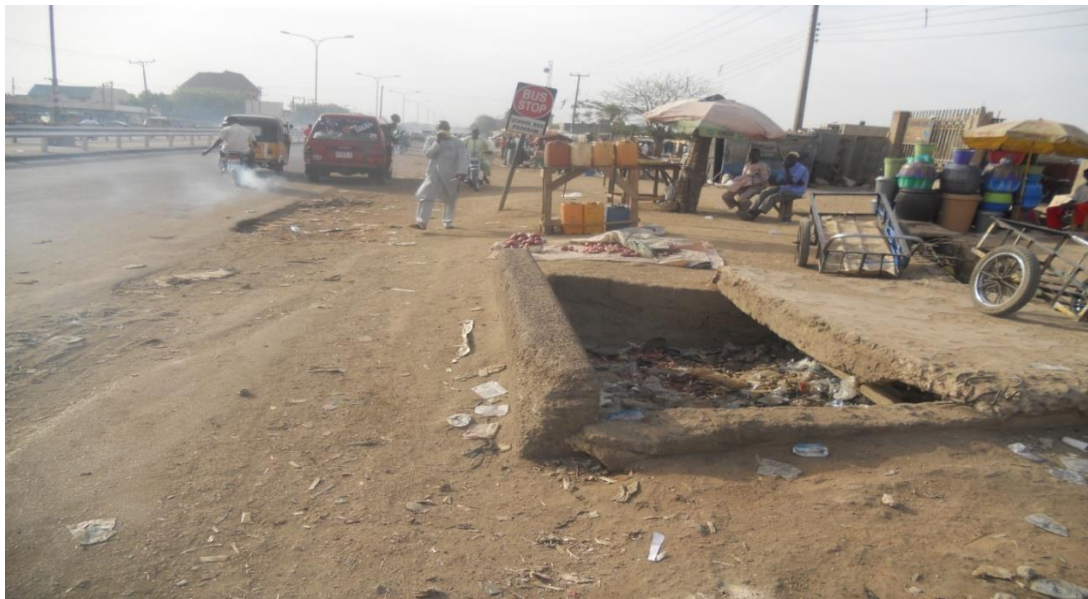
Figure 4.8 Improper drainages (Km 05+300) Airport Roundabout-Bachirawa Junction
