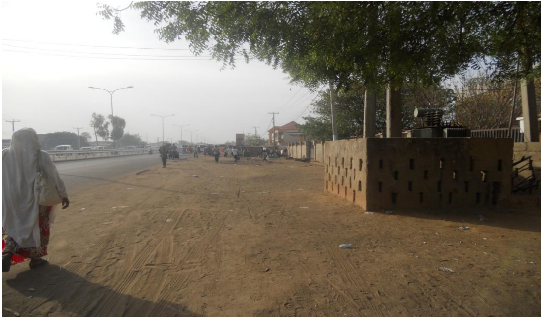
Figure 4.28 Improper transformer location (Km 07+700) Airport Roundabout-Bachirawa Junction
