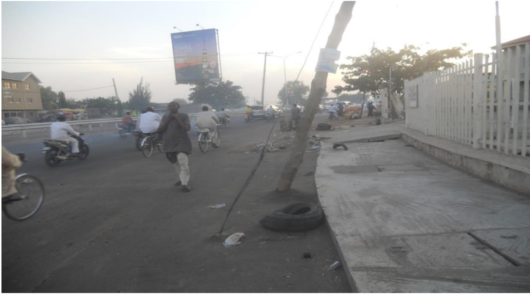
Figure 4.24 Improper pole locations (Km 00+40) Airport Roundabout-Bachirawa Junction
