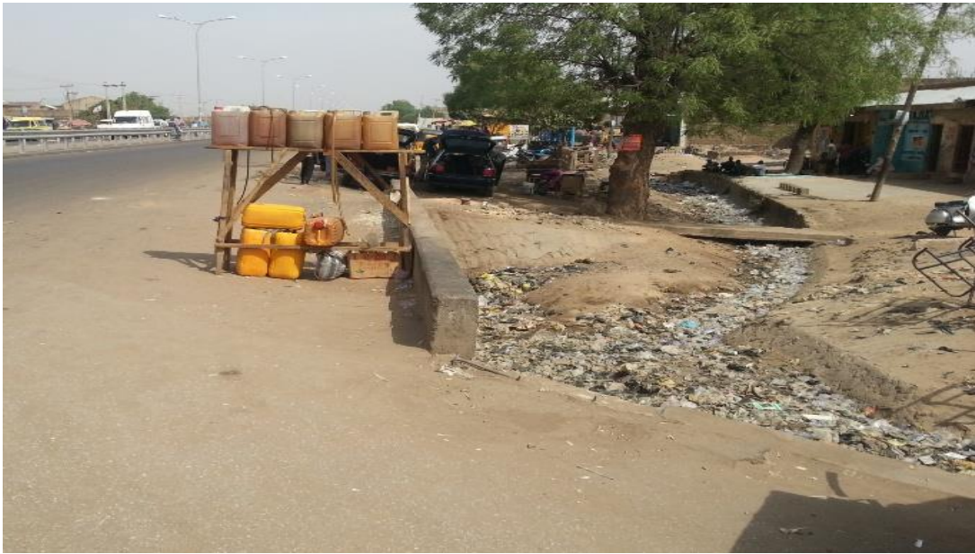
Figure 4.7 Improper drainages (km 04+250) Bachirawa Junction-Airport Roundabout
