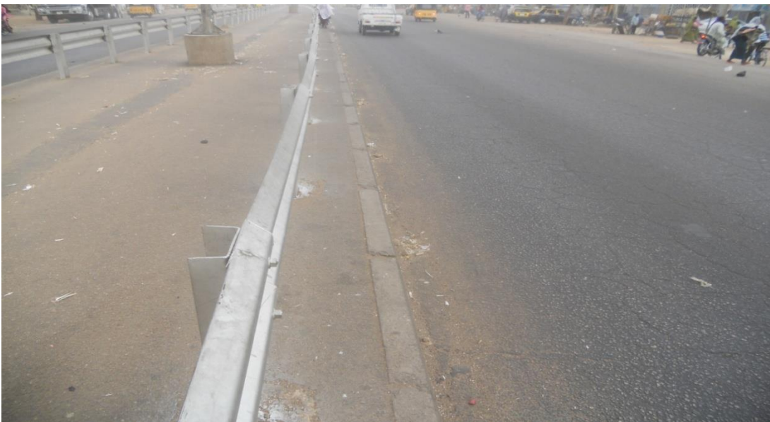
Figure 4.3 Absence of edge line markings (Throughout the road section)
