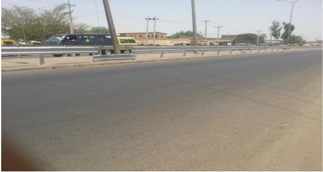
Figure 4.2 Absence of lane markings (Throughout the road section)
