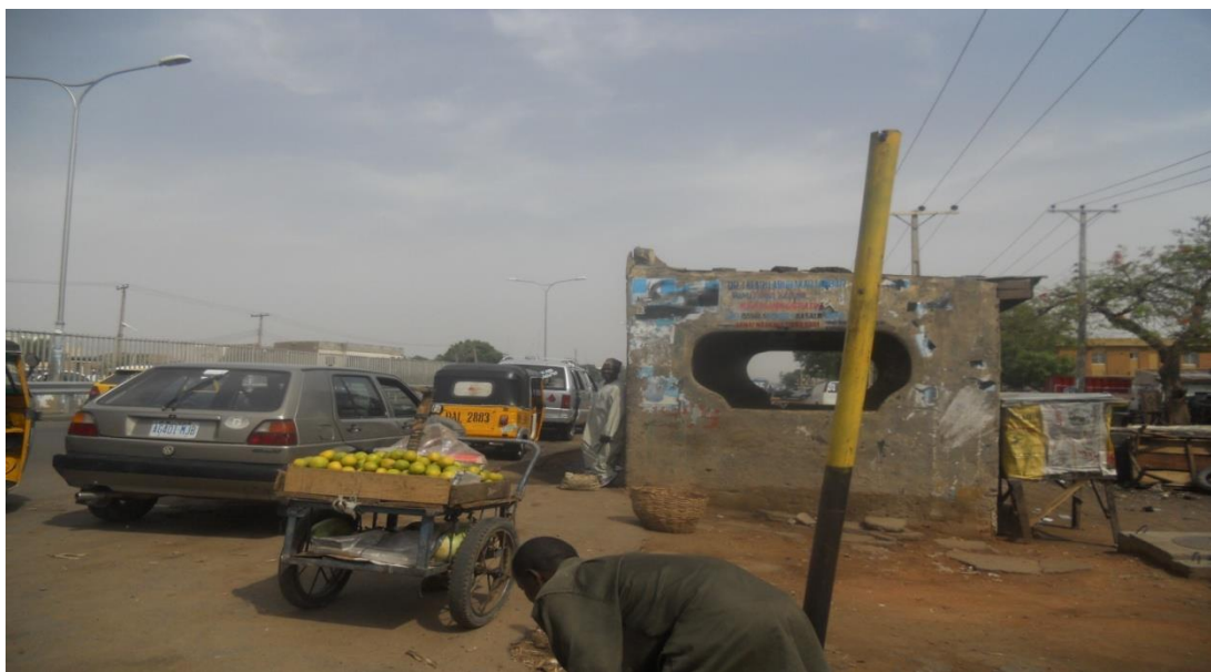
Figure 4.25 Improper bus stop shelter (Km 03+00) Airport Roundabout-Bachirawa Junction
