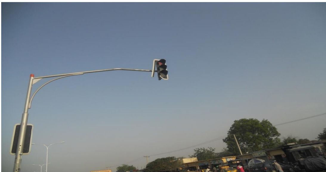
Figure 4.41 Damage and poor traffic signal head visibility
