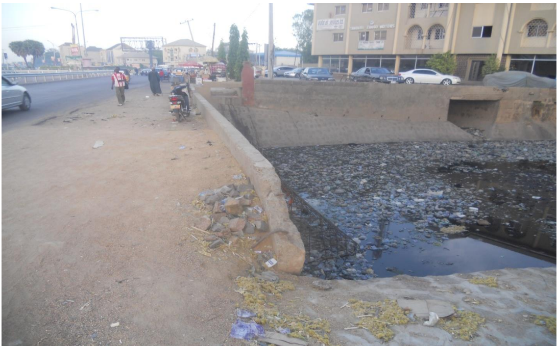
Figure 4.10 Improper channels (Km 07+700) Bachirawa Junction-Airport Roundabout
