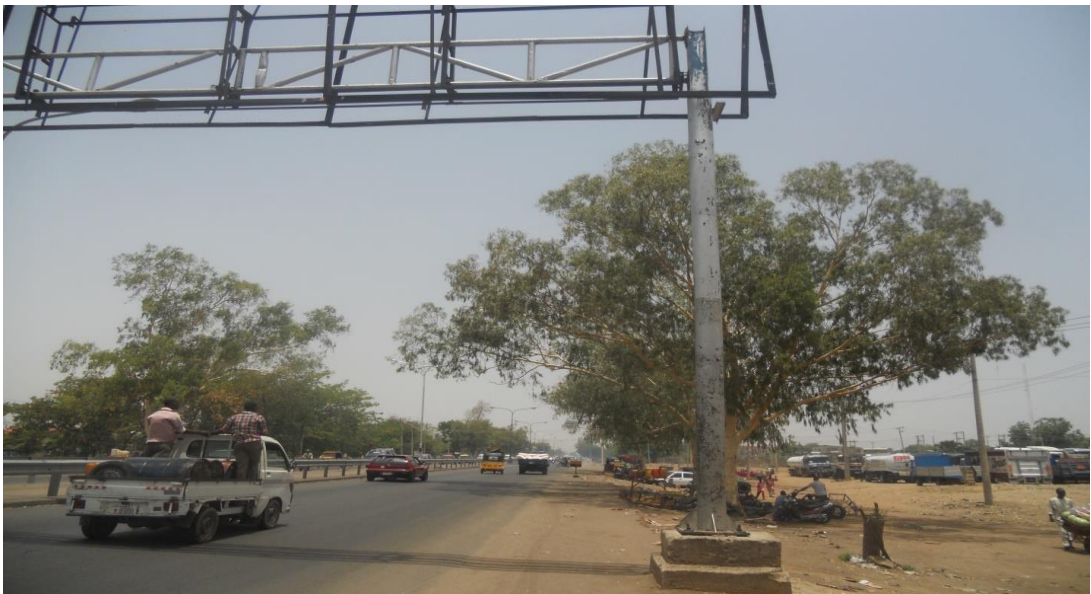
Figure 4.30 Improper location of advertising board (Km 00+550) Airport-Bachirawa Junction
