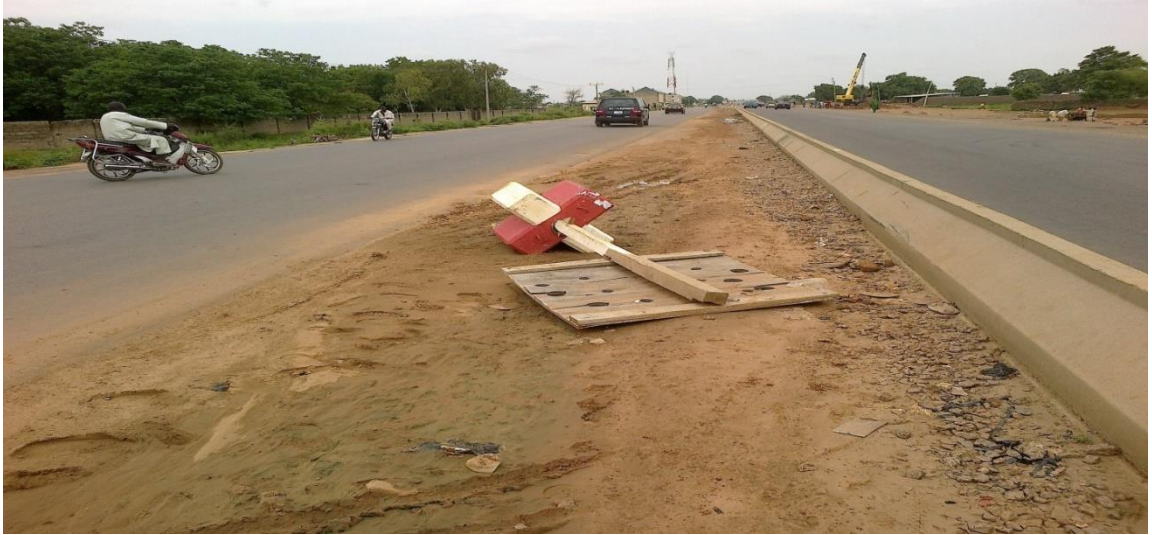
Figure 4-3 Damaged Warning Signs Km 5+100
