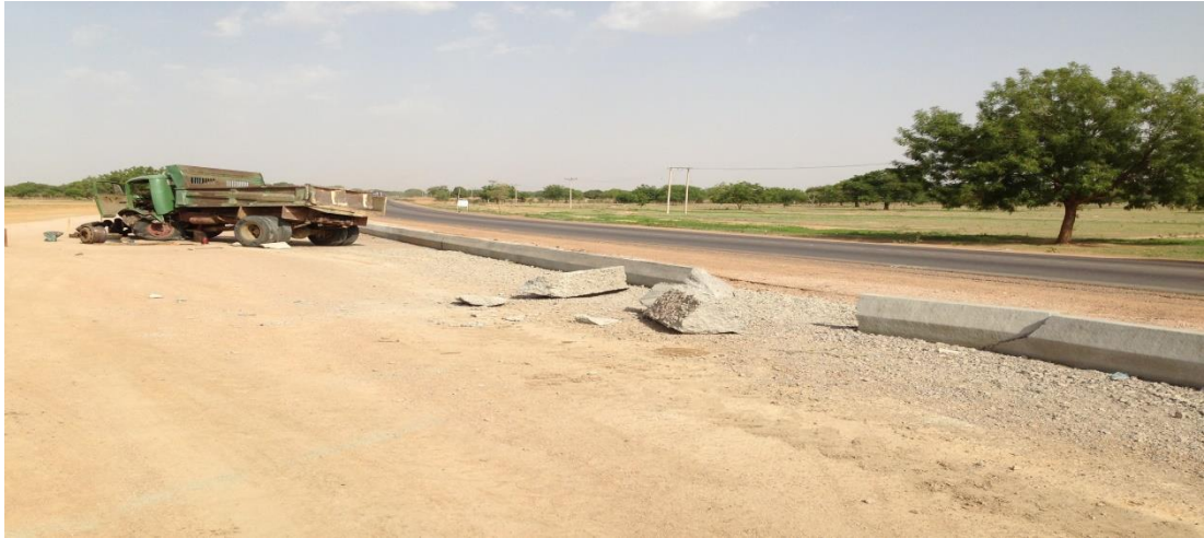
Figure D 11 Tipper Struck Median and Enters Working Area
