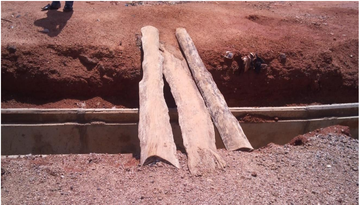
Figure 4-12 Dangerous Facility for Pedestrians 3+000
