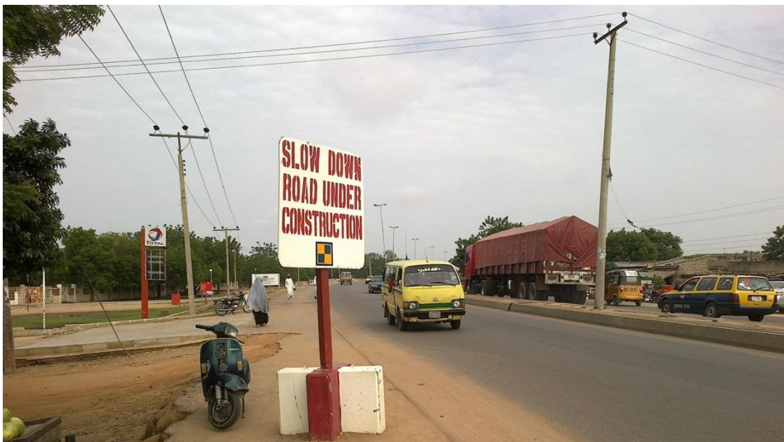
Figure 4-Error! Bookmark not defined. Wrong Sign Placement (100m before Work Zone)
