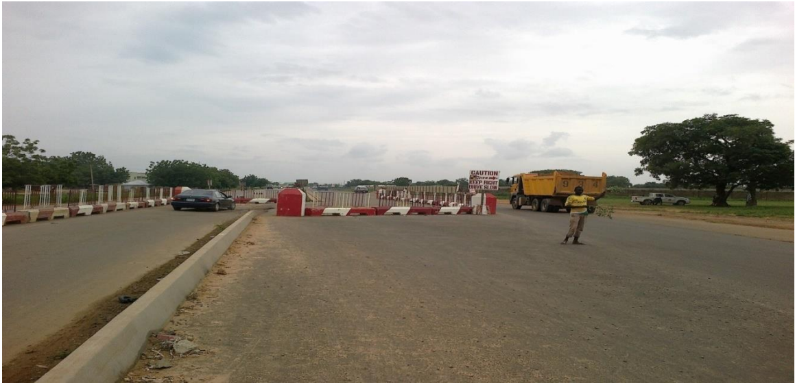
Figure 4-8 Dangerous Flagging Km 8+890
