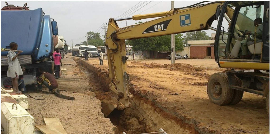
Figure 4-10 Unprotected Working Area Km 1+560
