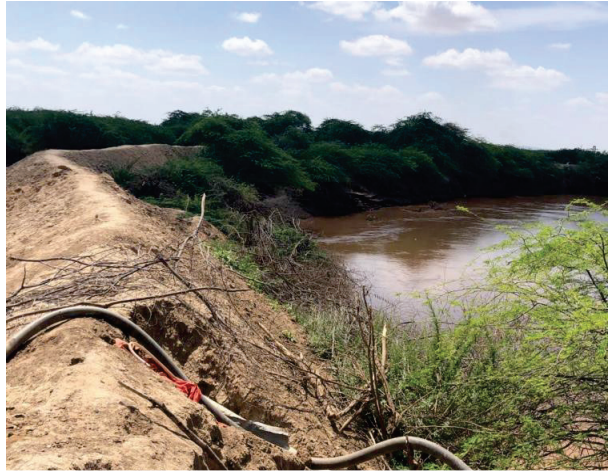
Figure 5.3 (a): Constructed Levees along the side of Shabelle River in the Study Area
