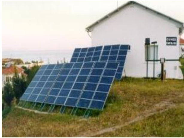
Figure 1.9 : Installed PV system for daily electricity (4,8 kWp) (EİE, 2011).
