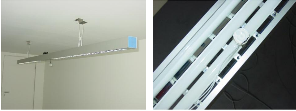
Figure 6.9 : The artificial lighting system and the photo sensor placement on the lamp with the connection of dimming ballast.
