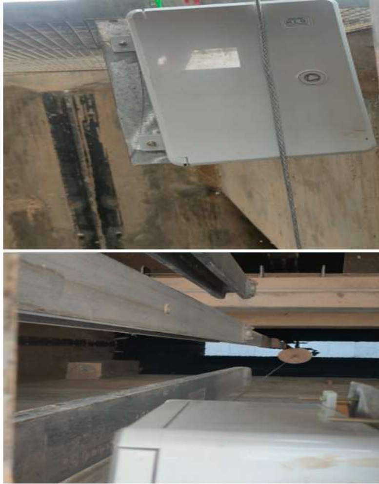
Figure 3.5 Tank level gauge
