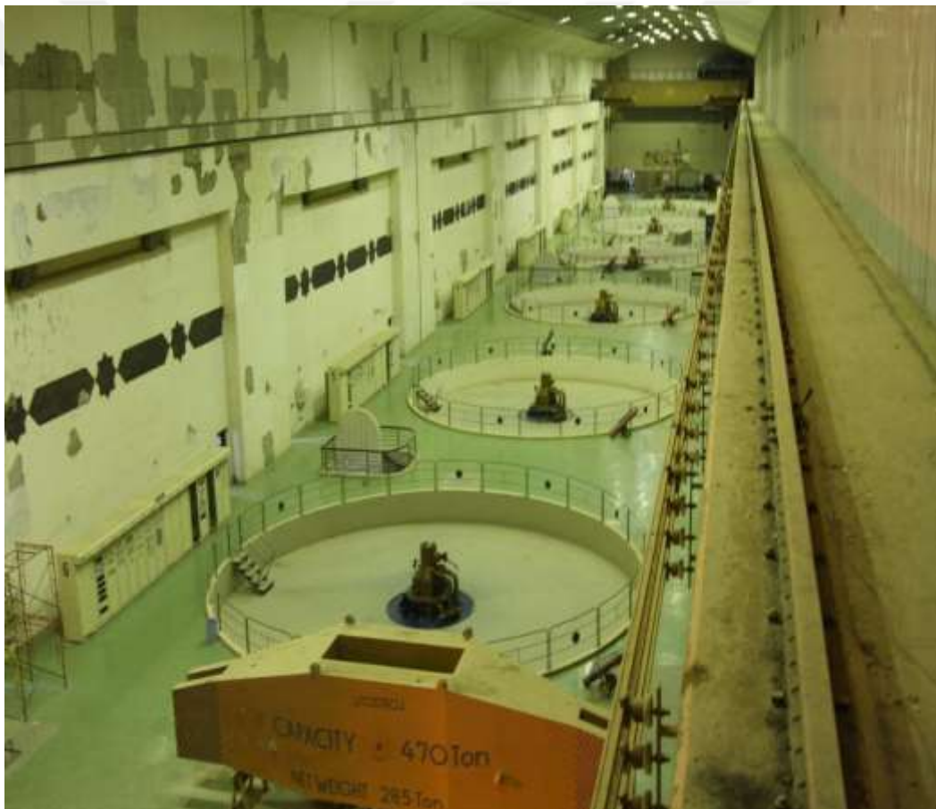
Figure 3.1 Overview of the turbine room inside the Haditha Dam, at Haditha, Iraq, Nov. 17, 2008
