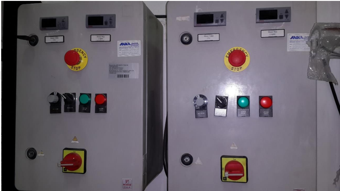
Figure 23. Control Panels of ROP and RPM Motors (for Motor Revolution Speeds)
