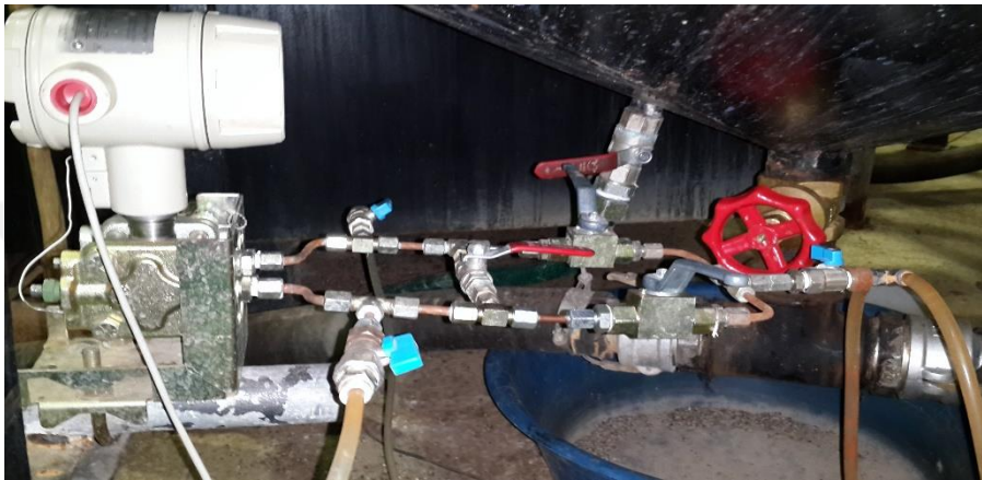
Figure 21. Lines from Test Section to Honeywell
