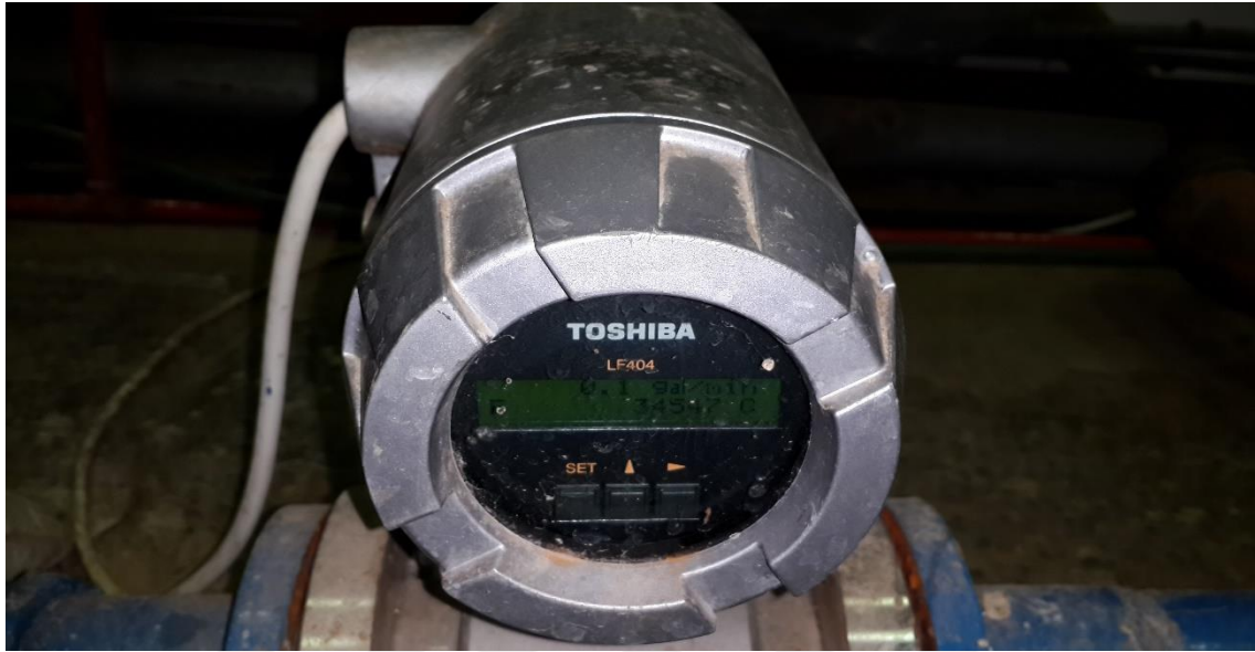
Figure 24. Toshiba Flow Meter
