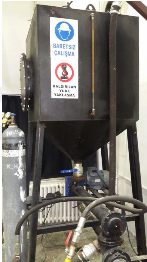
Figure 16. Cuttings Injection Tank
