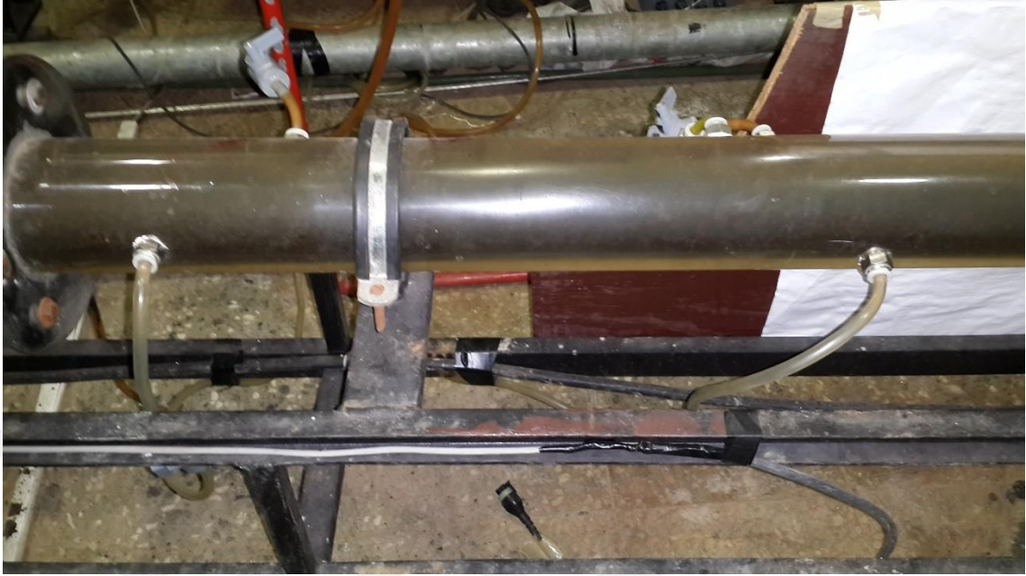
Figure 13. Lines Connecting to the Honeywell for Differential Pressure Measurements
