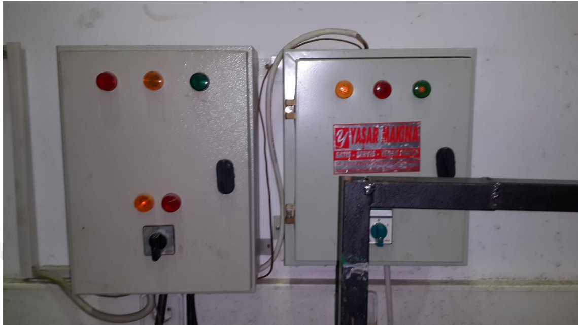
Figure 26. Pump Control Panels (On/Off)
