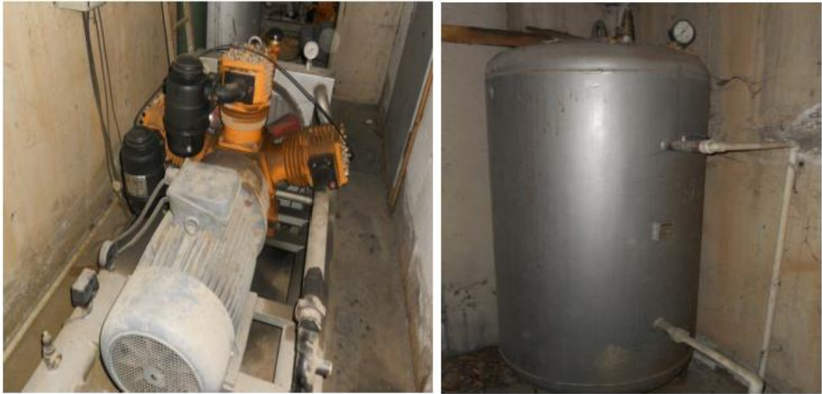
Figure 8. Gas Compressor and Accumulator Tank
