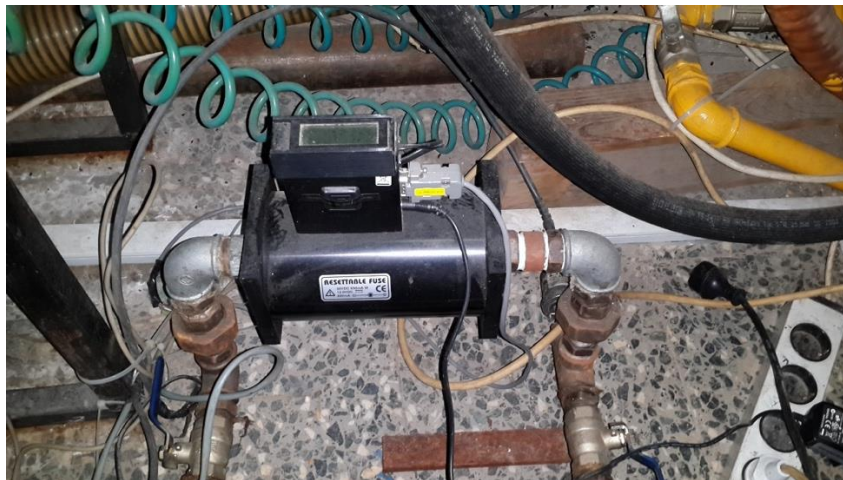
Figure 10. Dwyer Gas Flowmeter
