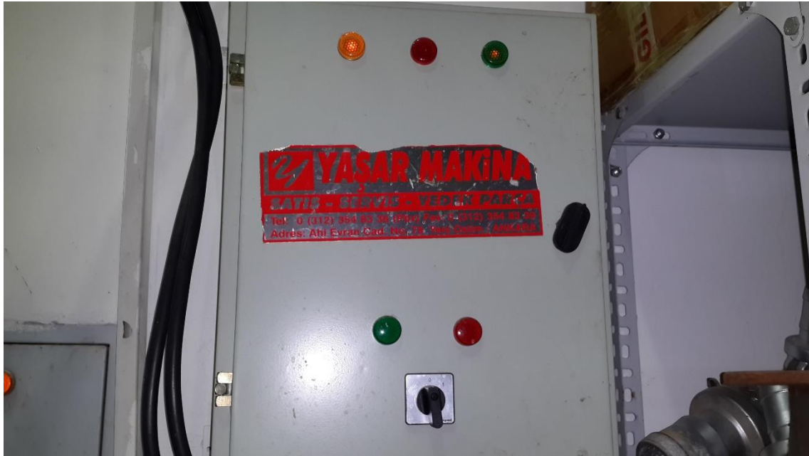
Figure 28. Mud Mixer Control Panel (On/Off)
