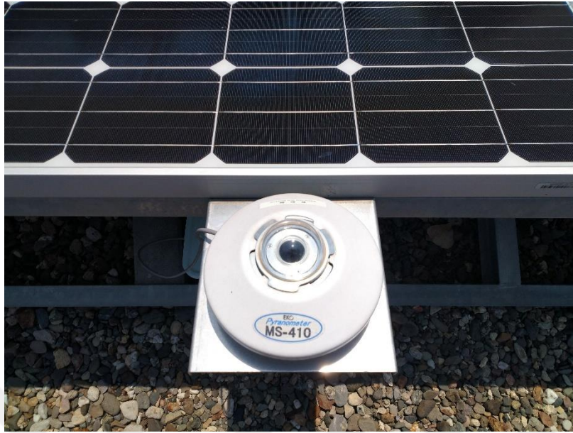
Figure 4-3. Pyranometer Used in Representative Site
