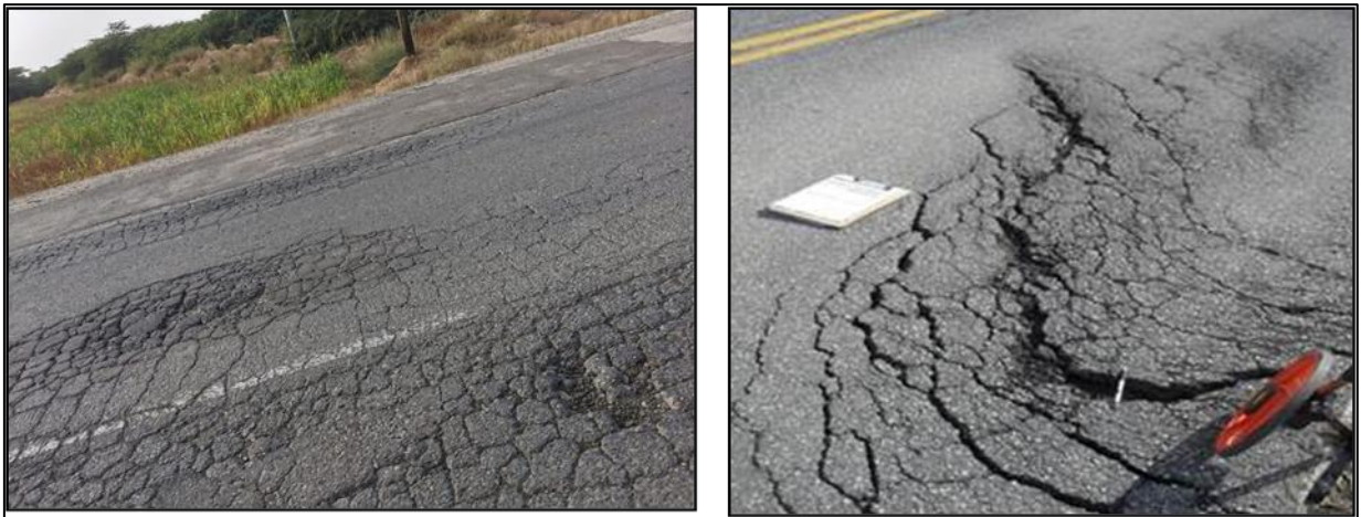
Figure 1.6: Cracks on Road [20].
