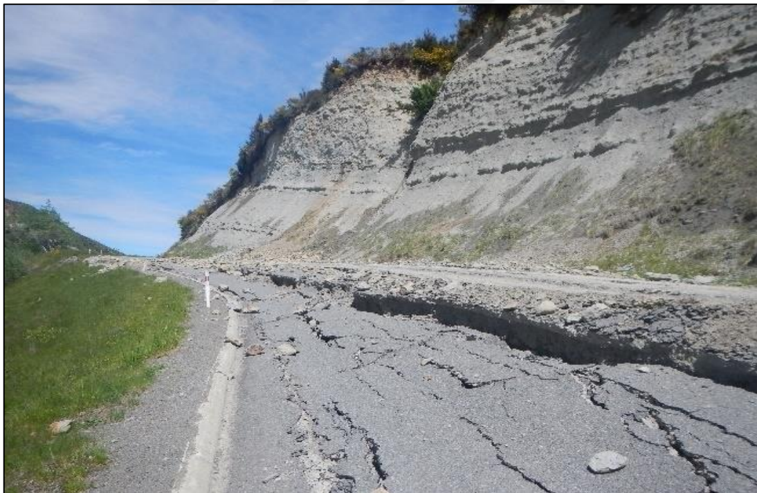
Figure 2.7: Settlement of Embankment Road [38].
