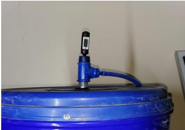
Figure 3.13: Cold Water Tank Pipe with Thermometer.
