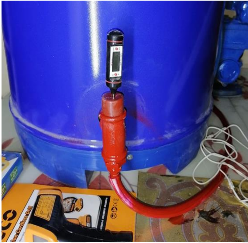
Figure 3.14: Hot Water Tank Pipe with Thermometer.
