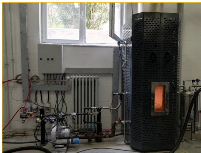
Figure 3.16: Flare system that disposes of the syngas obtained during pyrolysis tests.
