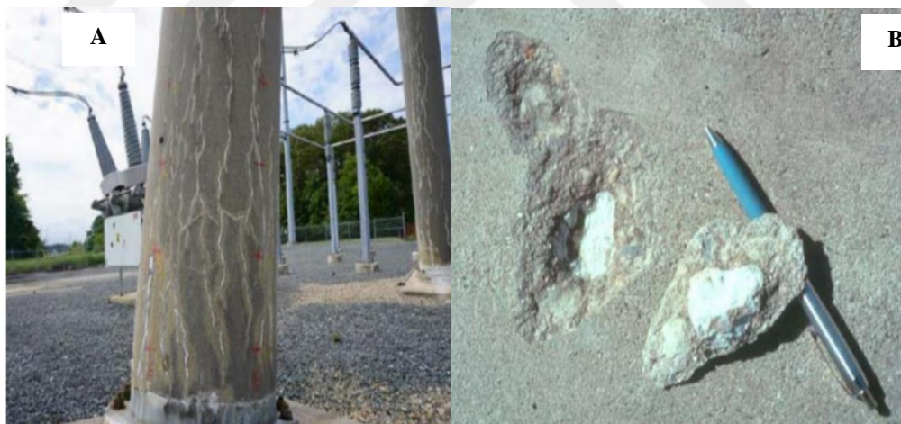
Figure 2.1 Crack produced by ASR, where (A) is map-cracking , and (B) pop-out cracking [28].
