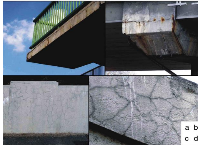
Figure 1.1 Map cracks in various places, where (a) shows cracks among the front, (b) head of the column destructed by the concrete spalling, (c) cracks all over the front side, (d) close view of the map cracking [5,6].
