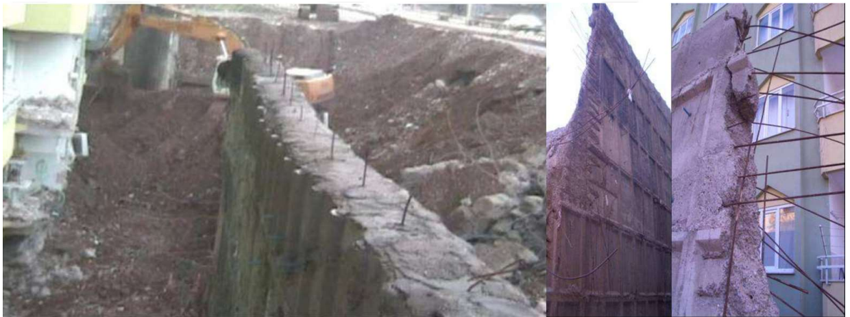
Figure 2.12. The pictures of wall failure and collapsed wall [13].
