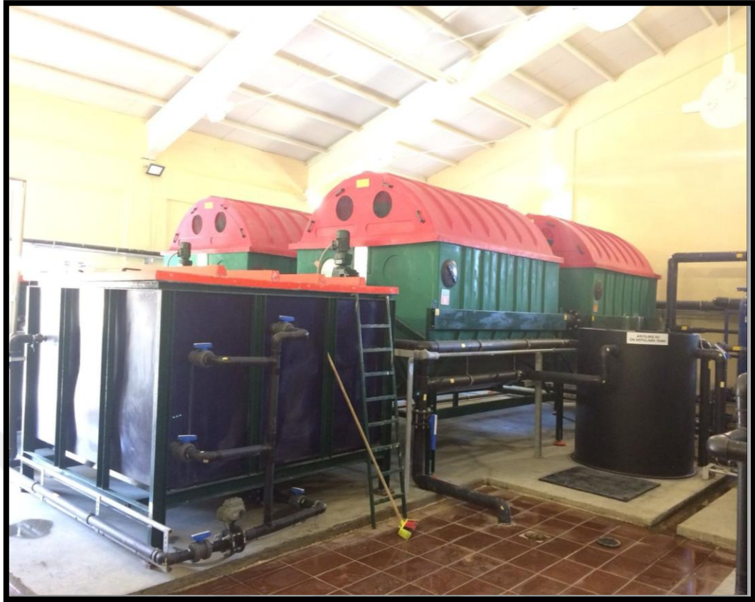
Figure 6.6. Wastewater treatment facility on Kilyos Campus.
