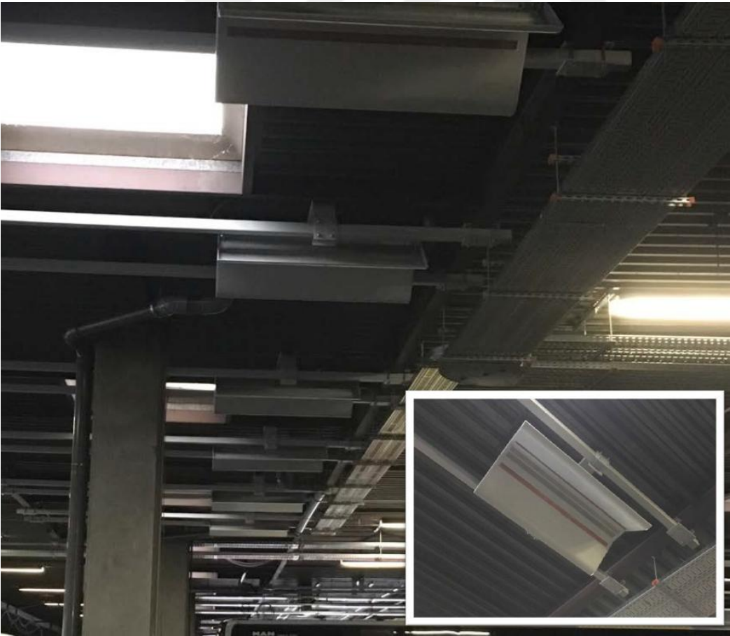
Figure C.2: Eindhoven depot indoor chargers.
