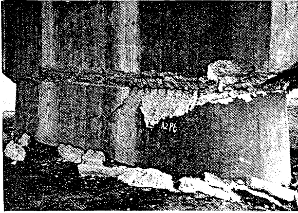
PHOTO B.3 Sendai Bridge, column damage. (Miyagi-ken-oki Earthquake of June 12, 1978), ATC (1979).
